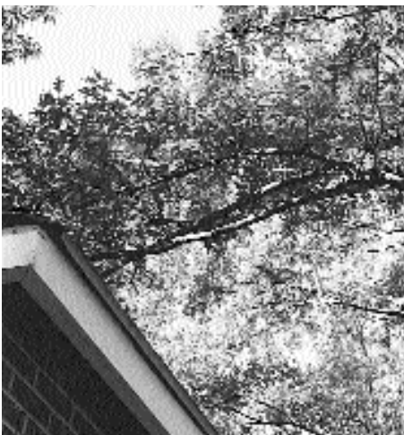
Prune all trees up to 6-10 feet from the ground and remove overhanging branches.
